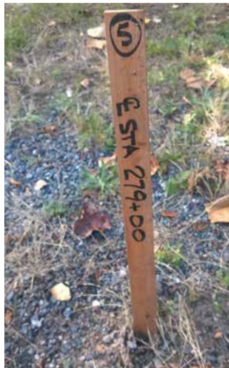
A project stake at station 279+00 to flag the location of a centerline cap.
