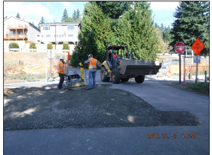
Driveway preparation for asphalt paving. Compaction application is being applied to the base course material.
