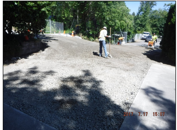
Completed installation and compaction of CSBC. This area is now ready for paving!
