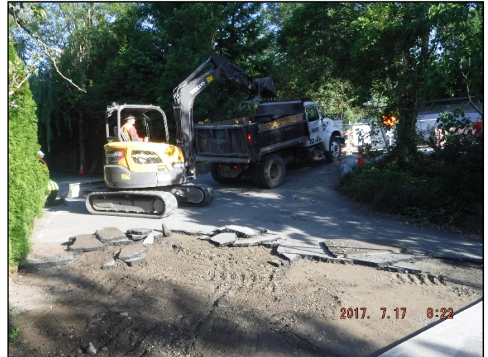
Asphalt removal prior to installation of Crushed Surface Base Course (CSBC) at a driveway approach
