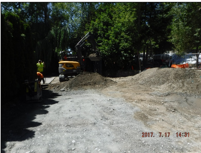
Contractor removing existing material at driveway approach before installing the CSBC base lift
