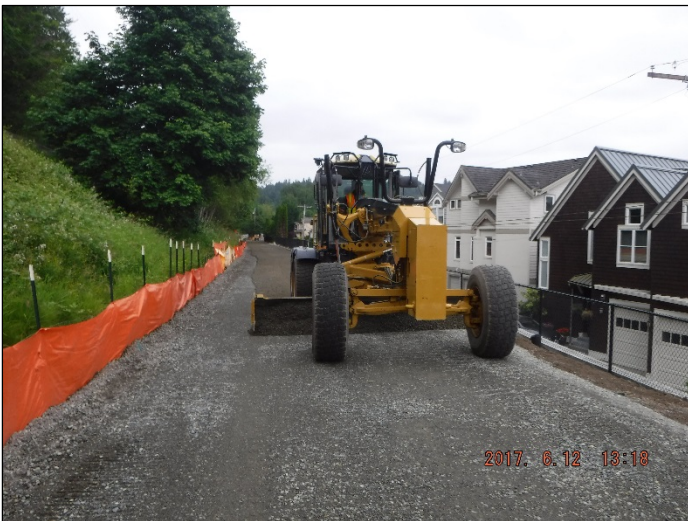
Continued fine grading of Crushed Surfacing Base Course (CSBC) for asphalt paving
