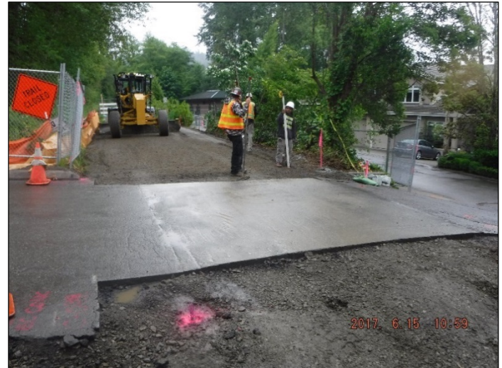
Continued fine grading of Crushed Surfacing Base Course (CSBC) for asphalt paving
