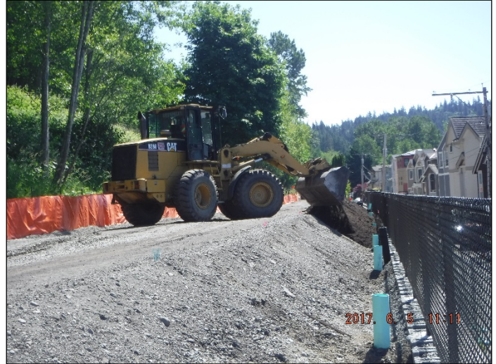
Installation of topsoil to the east side of the trail in landscaping locations
