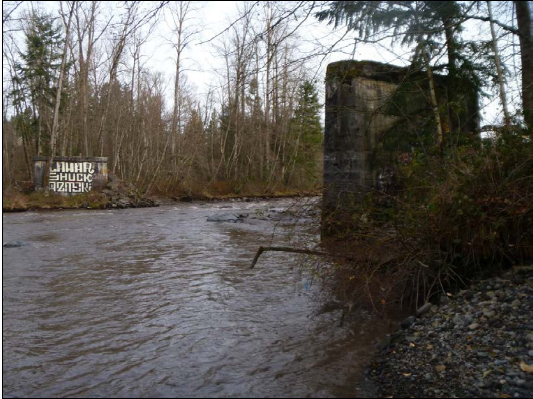
Photo 3: Proposed location of White River crossing over former SR 410 bridge piers, facing northeast
