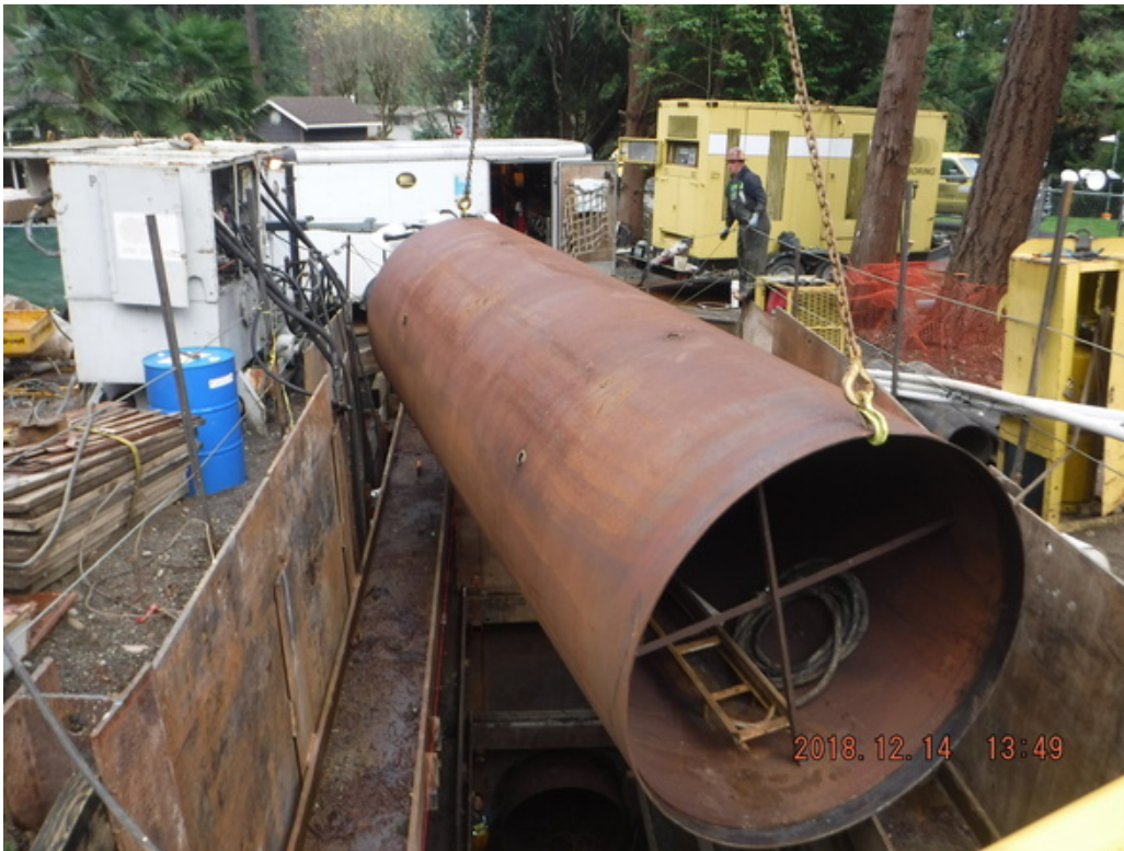
A segment of pipe being lowered into the pit for installation. The pipe is six feet wide.
