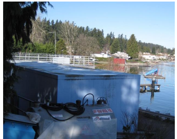
Current Sunset Pump Station generator enclosure (shows existing color)
