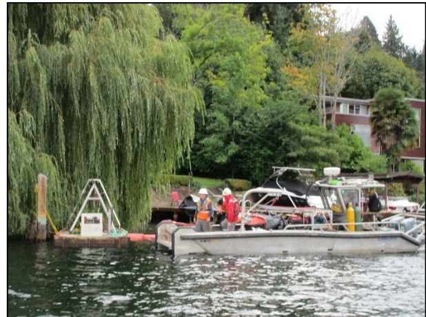
Crew members working from a dive boat that powers a hose used to expose underwater structures.
