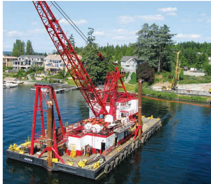
Crews worked from a barge this summer to gather information about alignment conditions
