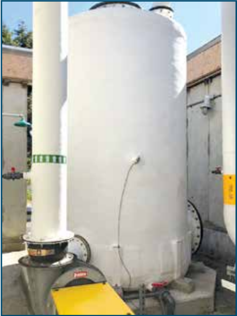
Example of a carbon filter used in some odor control systems.
