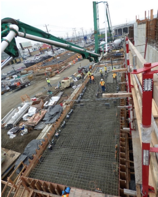
Crew members pour over 265 cubic yards (53,523 gallons) of concrete at the treatment station's future electrical building site.
