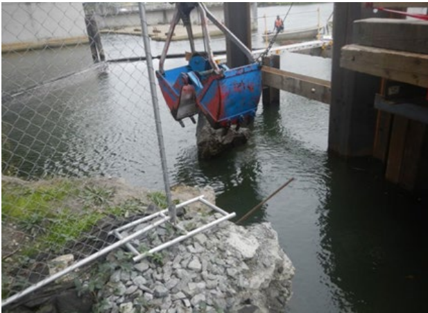
Concrete debris are removed from the Duwamish River at the outfall project site.
