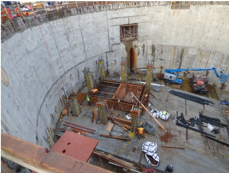
An inside look at the Equalization Basin – an underground tank that will be a key part of the water treatment process at the Georgetown Wet Weather Treatment Station.
