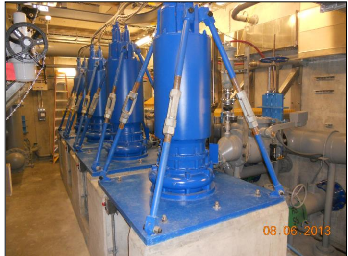
The new pumps in King County's Kirkland Pump Station are now operational.
