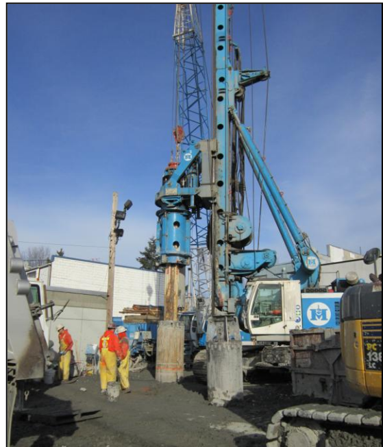
Equipment, similar to this, will be used to install piles at the Kirkland Pump Station.
