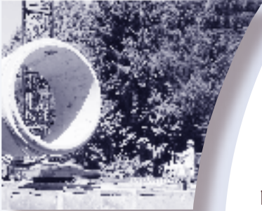
Workers guide a pipe section as the crane lowers it into the trench.
