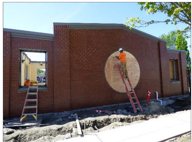
The odor control facility is almost ready for the project art.
