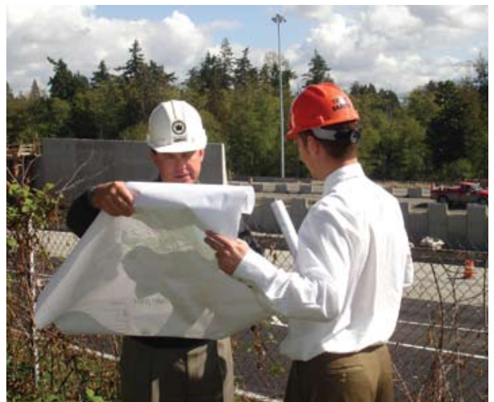
Pete reviews plans to increase highway capacity along I-5 in south King County.
