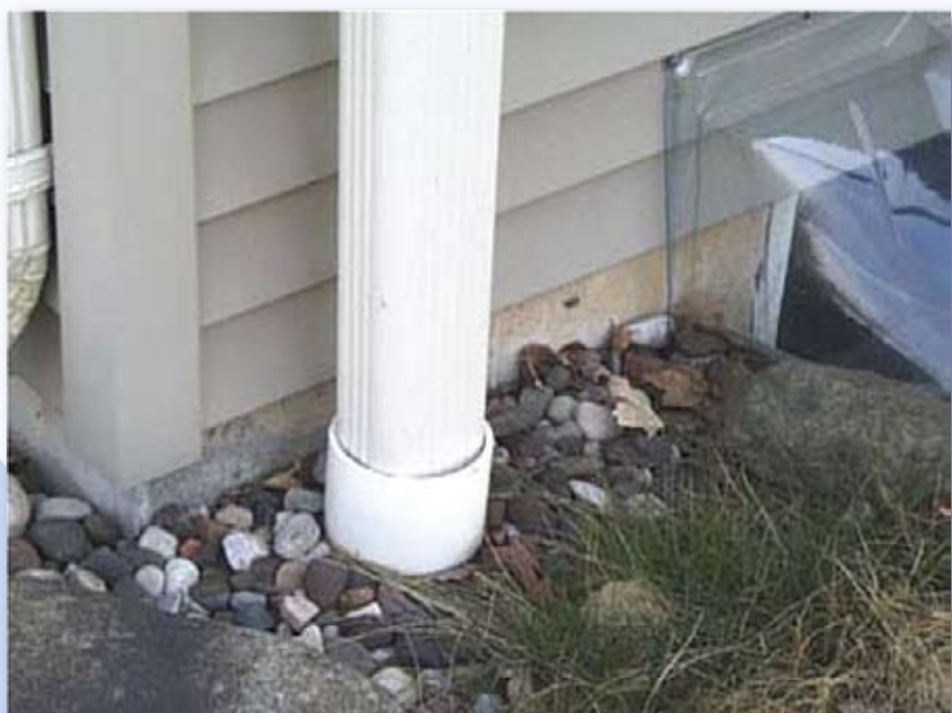
Downspouts are directly connected to combined sewers in older cities like Seattle
