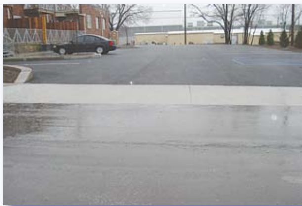
Permeable asphalt in the parking area (above) allows rain to soak in the ground underneath. On the street, rain runs off into the stormwater or combined sewer and stormwater system.
