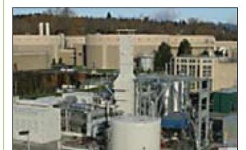
Fuel cell and digesters
