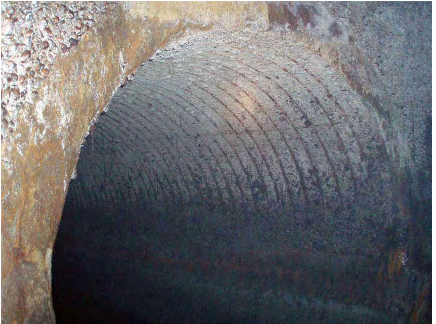
Corrosion has exposed rebar and aggregate on the inside of the North Interceptor
