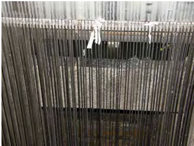
Current West Point bar screens. Note variance in spacing between bars
