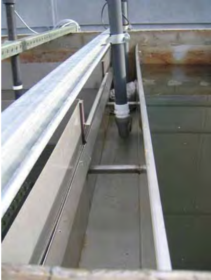
Chemically Enhanced Effluent Weir
