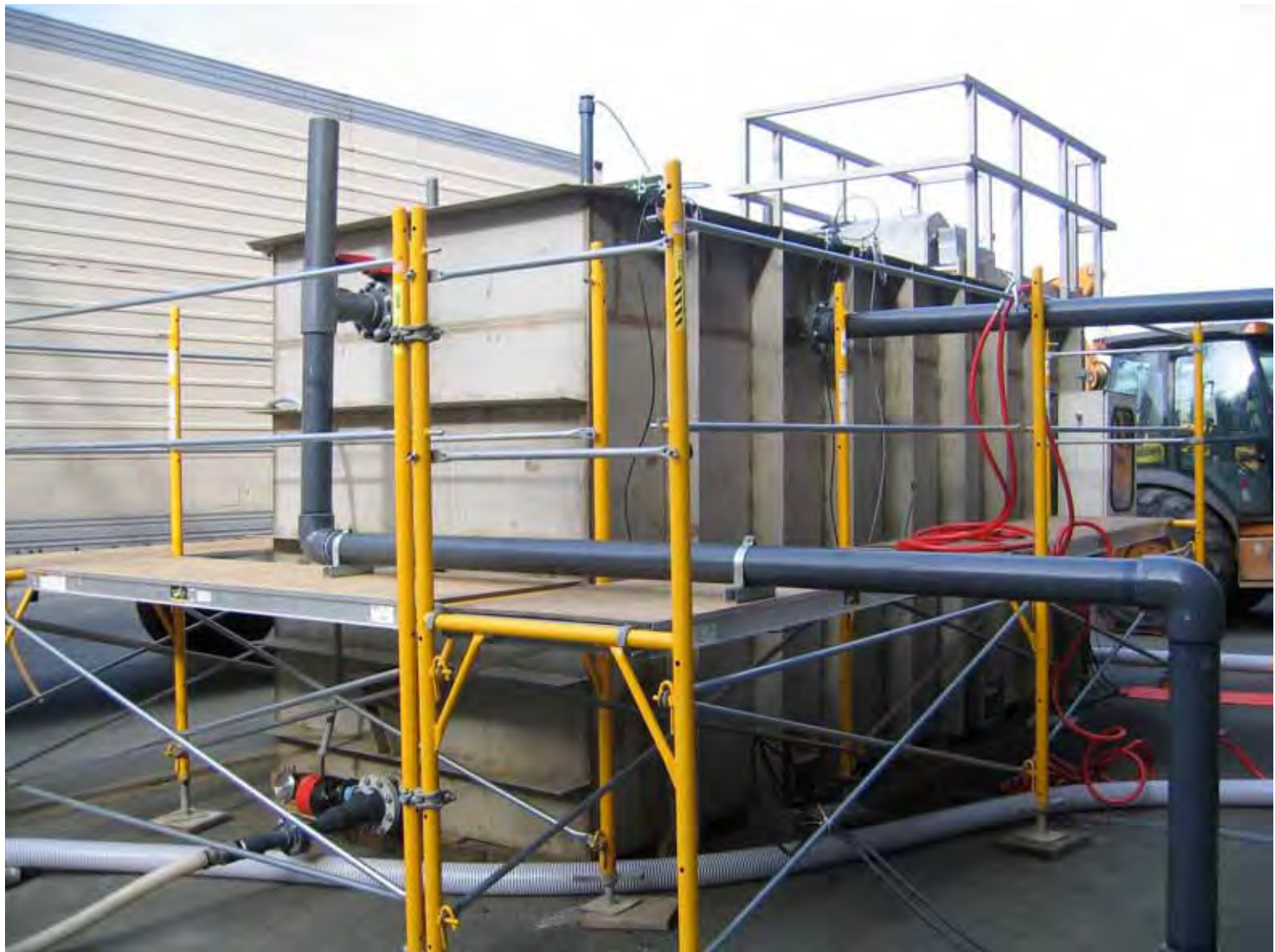
CSO Treatment Pilot Plant Exterior
