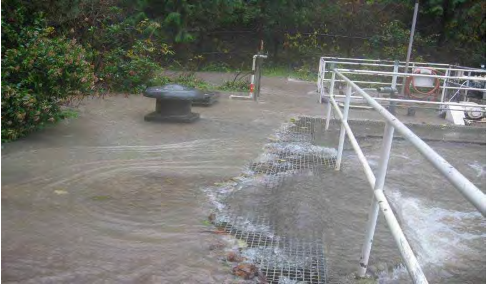
Urban flooding – Carkeek CSO Treatment Plant
